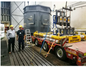
The three-phase 11kV, 20MVA pmFCL undergoing performance testing.
